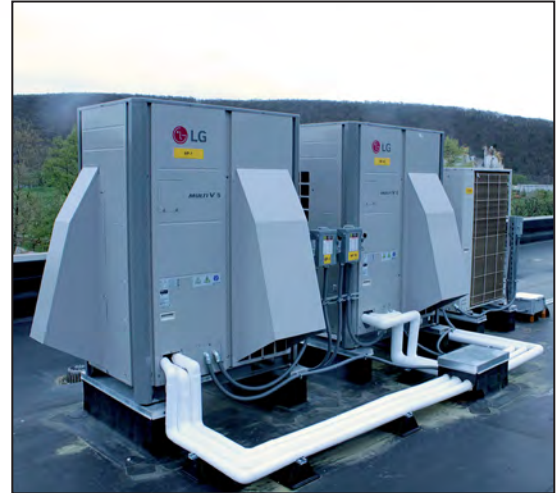
ABOVE: Two of the new energy efficient VRF heat pumps installed on the library building roof in 2020; part of the library's $1.3 million Green HVAC project. The new system includes MERV 13 filtration and state of the art in-duct UV disinfection. The project was funded in part by the New York State Construction Aid for Libraries Program.
