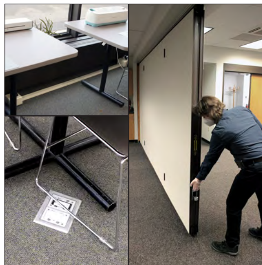
The library completed several New York State funded health & safety upgrades in 2021. Top, left: these included replacing loose wiring and outlets in the Creation Station with fixed raceway electrical outlets. Bottom, left: eight raised electrical floor boxes were replaced with recessed receptacles. Right: a new Community Room folding partition replaced a worn out partition. Other improvements included security system and fire safety system upgrades.
